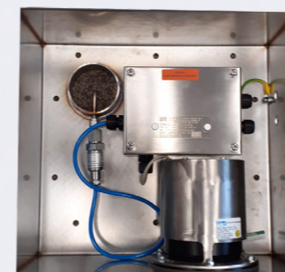
> PP14 (OUTLET UNIT) INTERNAL COMPONENTS
